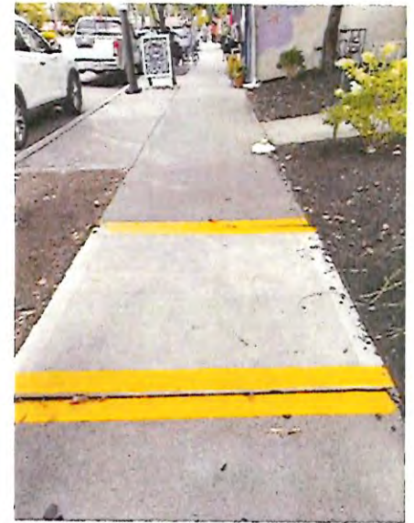
Xenia Ave sidewalk issues
