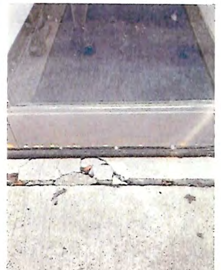
threshold needs repaired Gym Entrance
