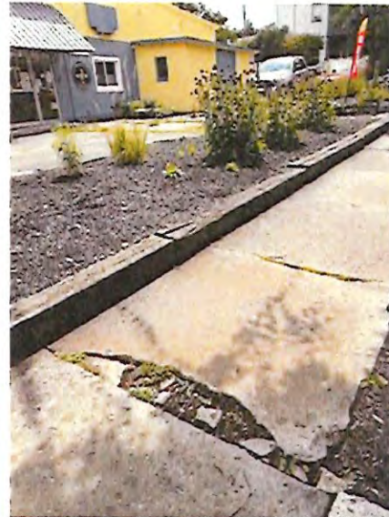
Dayton Street sidewalk issues
