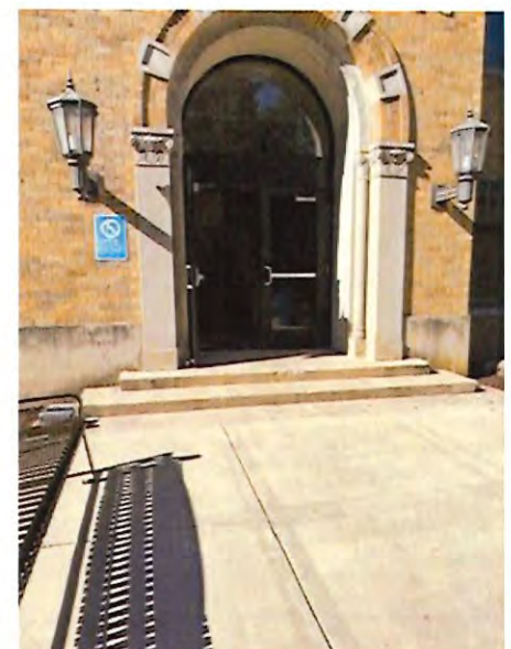
Front Entrance needs railing
