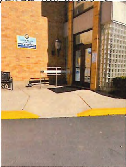
Bryan Center Main Entrance curb cut 3ft 7inches slop grade to steep
