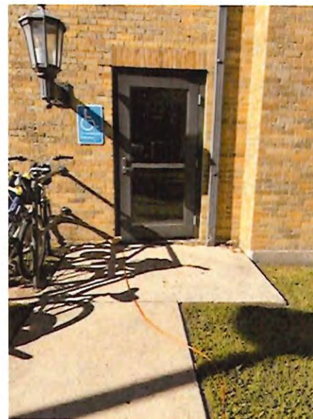
threshold needs ramped Gxn Entrance
